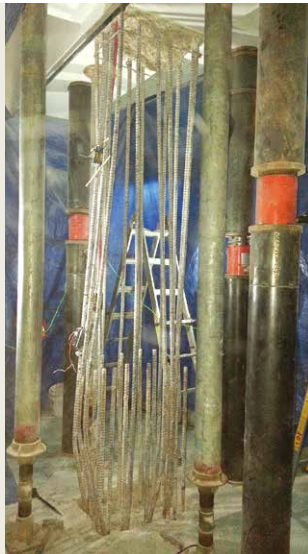
Vertical steel bar buckling
