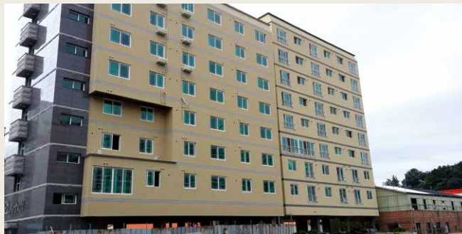
Two buildings are shown distortedly due to column punching settlement.
