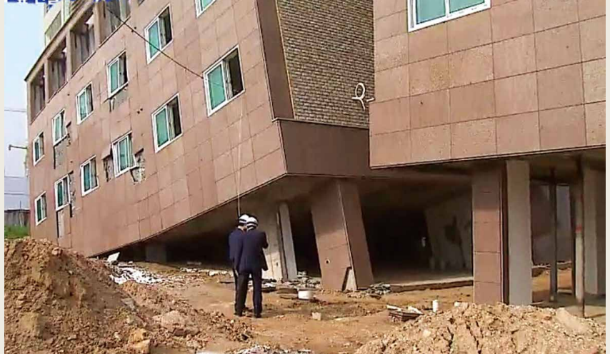
No settlement occurred in the first floor foundation, but punching failure at the column supports caused the structure to tilt.
